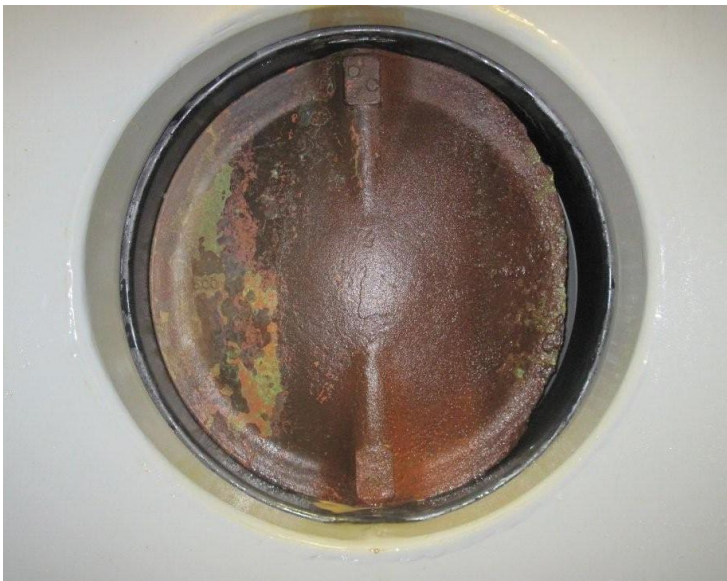
Figure 2: Example galvanic corroded disc
